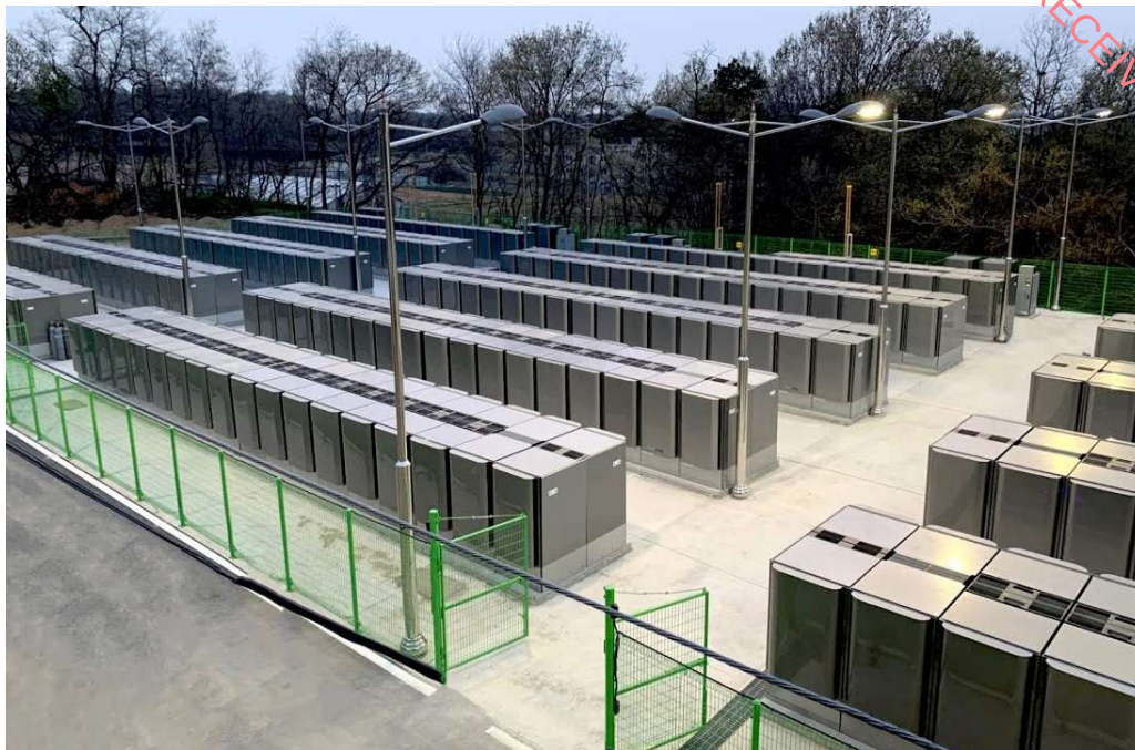
Figure 2.20 Modular Energy Servers positioned at ground level 9
